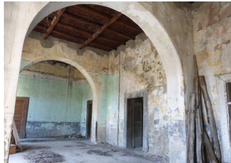
Fig. 7 The main room of the Noble Floor before restoration design (Luciana Di Gennaro, 2016).
