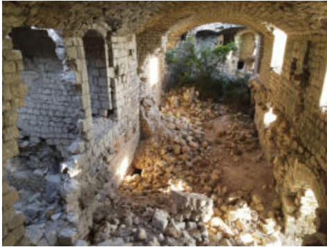
Fig. 11- Inside of the barracks, view from the northern wing into the main tract (the wall part in the upper left corner recently collapsed) (photo by Ivan Vratnica, 2020)
