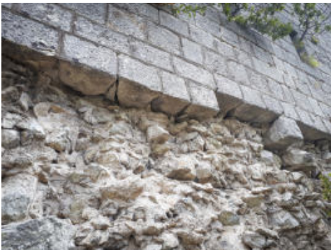
Fig. 6- Visible wall structure after devastation (photo by Ivan Vratnica, 2020)
